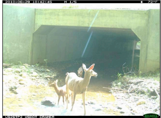
Figure 4. Concrete culvert under US 101 in Washington with black-tailed deer doe and fawns © P. Cramer, J. Kintsch, & WSDOT
