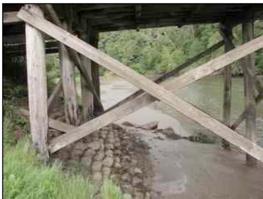
Figure 22. Bank under structure on north side
