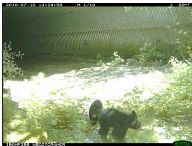
Figure 15. Black bear cubs passing through culvert behind mom, under I-90 Washington © P. Cramer, J. Kintsch & WSDOT
