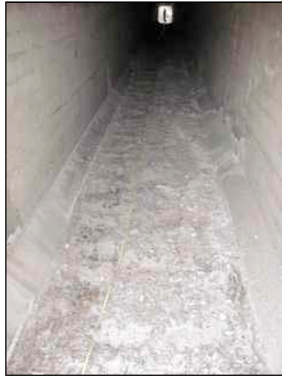
Figure 63. Long, narrow tunnel effect
