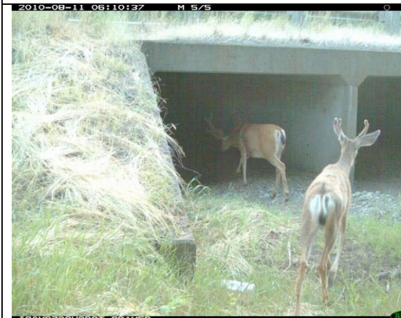
Figure 104. Mule deer bucks entering and using culvert on I-90 MP 73.
