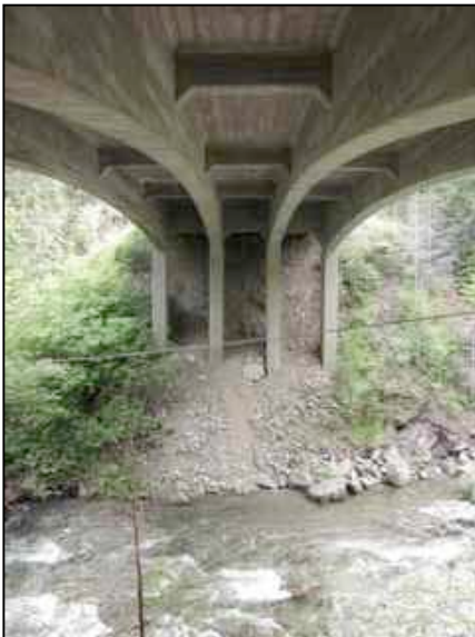
Figure 59. Steep bank on west side
