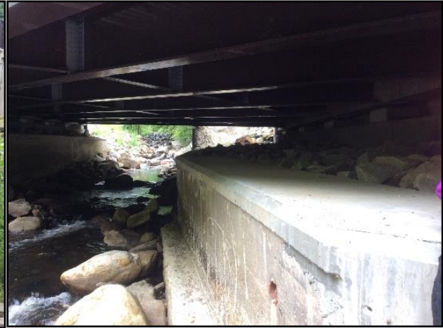
Figure 57. Four dry passage options under bridge in Becket, MA. At the highest level, concrete and riprap passageways are available for wildlife use. Below, a narrow concrete ledge and nearby boulders also offer dry passage.
