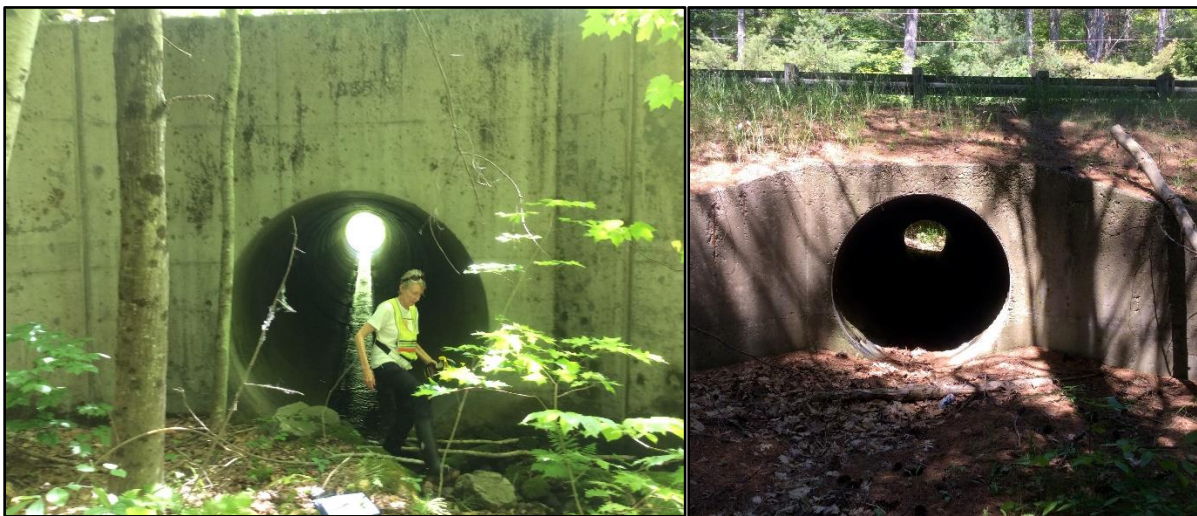
Figure 11. Circular culverts provide full or partial dry passage for terrestrial wildlife. The culvert at left could functionally pass large mammals, such as bear. The culvert at right is smaller in diameter (5 feet), which is still large enough for many species.
