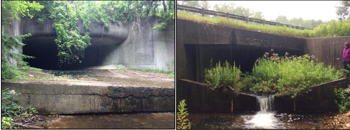
Figure 14. Outlet drops at culverts on I-90 near mile 12.4 (left) and mile 13.7 (right).
