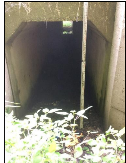
Figure 58. 4.7 foot tall culvert under Route 7 near New Ashford, MA. Black bear tracks filled this passageway.
