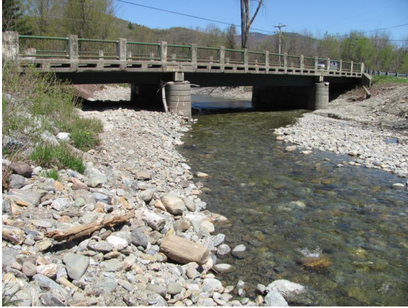
Figure 13. Route 118 bridge over Trout River in Montgomery, VT looking north from West Hill Road. (photo: Bob Hawk, 5/7/12)
