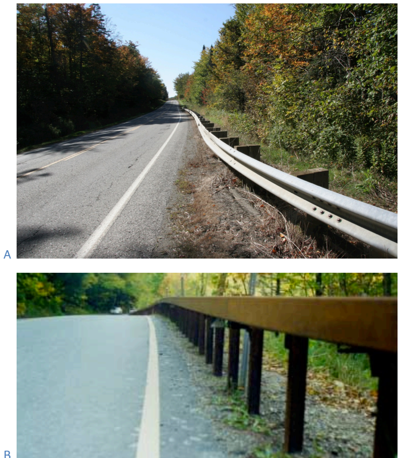
Figure 16: Guard rail types. A) W-beam guard rail separating a highway in the Green Mountains from wetland-forest habitat (to the right). B) Box-beam rail in forested habitat (VTrans, 1999).
