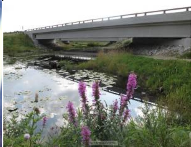
Dry pathway installed through riprap slope under a bridge in Minnesota ©P. Cramer
